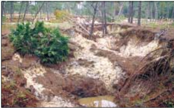
Figure 19. Human-induced sinkholes formed during the development of an irrigation well affected a 20-acre area and ranged in size from less than 1 foot to more than 150 feet in diameter. (Photograph courtesy Ann Tihansky, USGS.)
