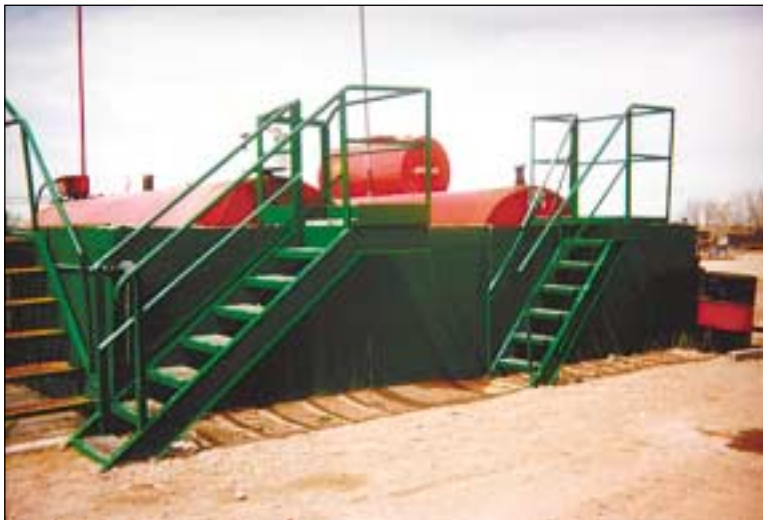
Figure 17b. Properly constructed containment facilities can protect the aquifer from potential fuel spills. (Photograph courtesy Lafarge.)
